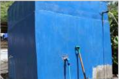
Water Tank (After)
