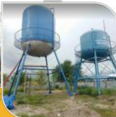
50 CU.M. ELEVATED STEEL TANK AT PS NO. 18, PRK. LOWER SHUTTLE, VARBC, BRGY. SAN JOSE
